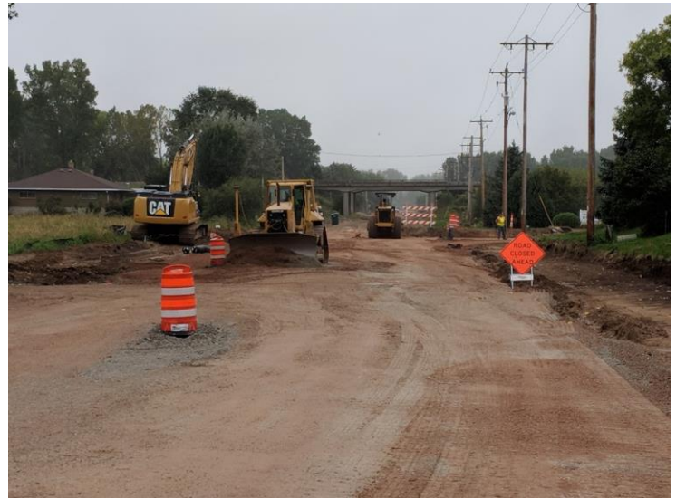
RC Excavating placing aggregate base on N. Gillett Street North of Evergreen Drive
