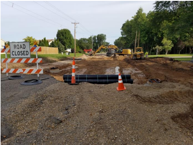
RC Excavating digging down to subgrade (both photos are from previous week work)
