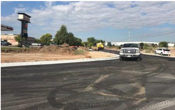
New curb and gutter as well as lower layer of asphalt on the SW corner of Victory Lane and Casaloma Drive
