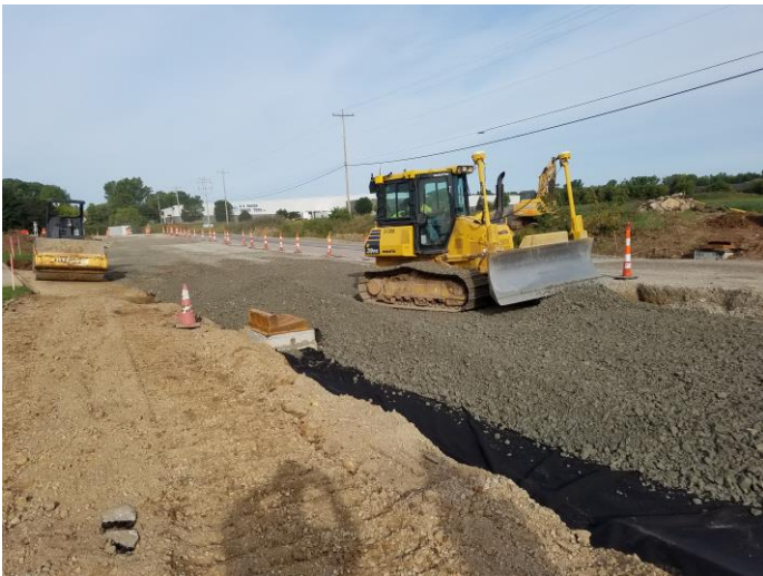
Relyco placing road base at the Victory Lane Roundabout West of Casaloma Drive
