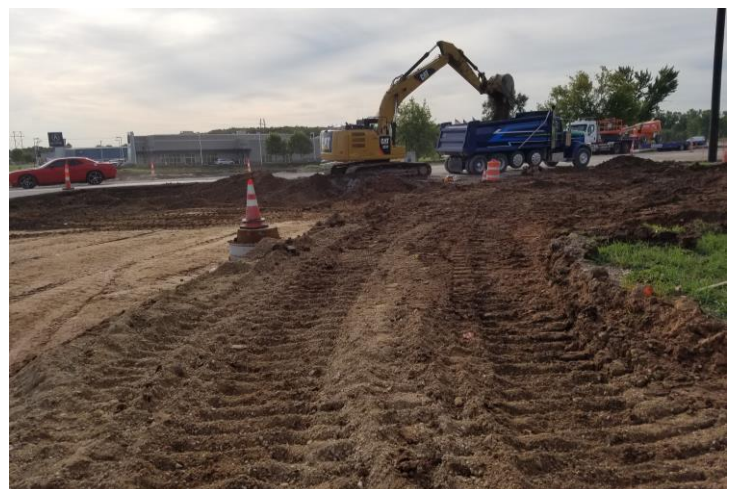
Relyco excavating road base at the Victory Lane Roundabout South of Victory Lane on Casaloma
