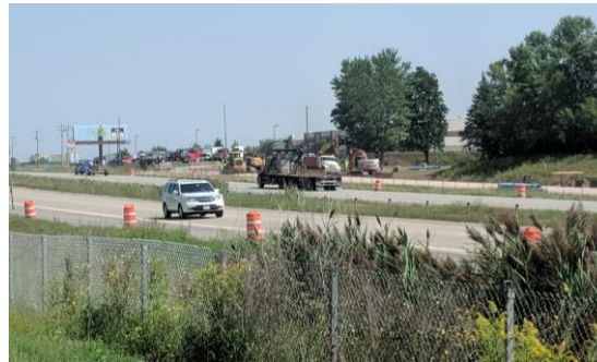
View from Mid Valley Drive Looking north east at construction across I-41
